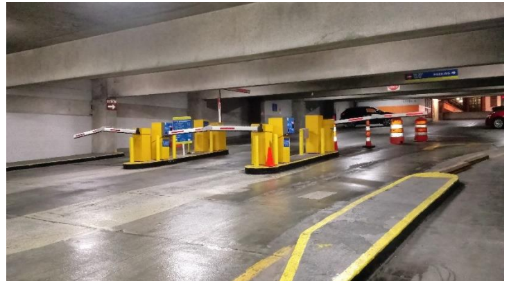
Figure 8 - PARCS Equipment (Victorian Square Garage)
